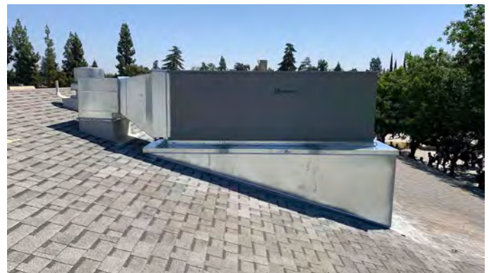
Bullard High School Kitchen Hood, Fresno Unified School District
