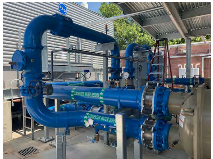
Sanger High School Central Plant, Sanger Unified School District
